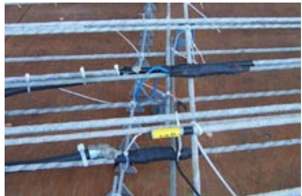
Red River Bridge: Fibre Optic Sensors for Structural Health Monitoring System
